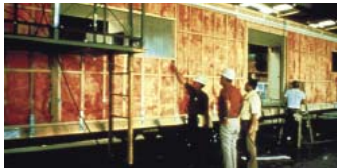
The HUD Code sets stringent performance standards for structural framing, heating and air-conditioning, plumbing, thermal, and electrical systems.
